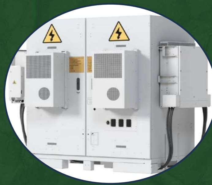
Battery Energy Storage as a Service Storage of electric energy stand alone or connected to Photovoltaics
