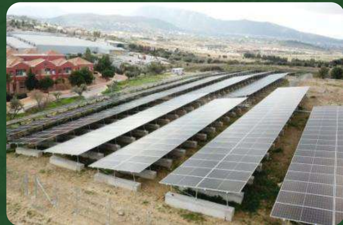
Pierce – The American College of Greece (East Campus) 499KWp
