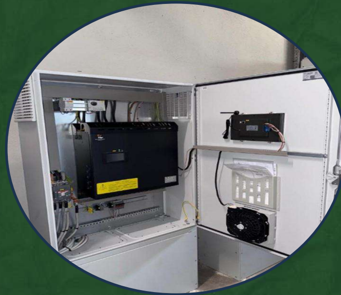
Power Quality as a Service Power Quality Improvement with voltage stabilization and harmonic distortion filters
