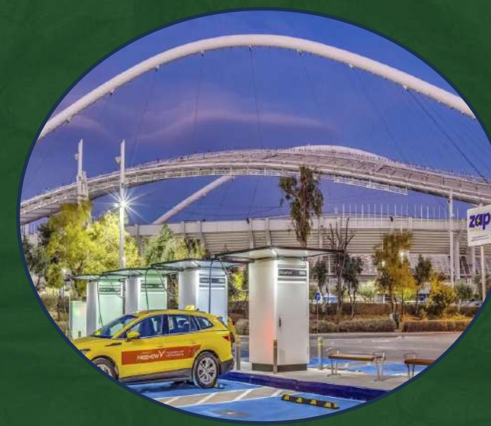
Electric Charging as a Service Application of Electric Charging Systems for cars and other vehicles
