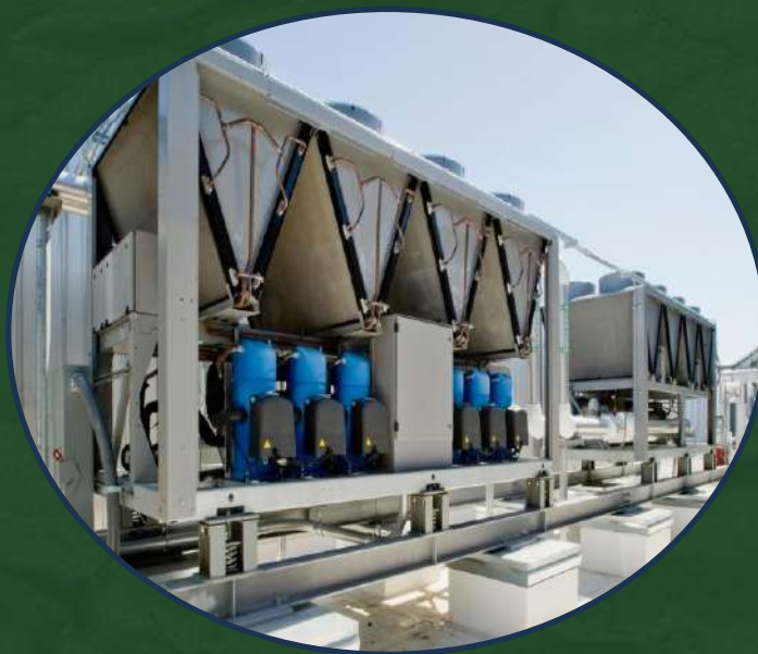
HVAC-R as a Service Upgrading of Heating, Air Conditioning, Ventilation, Commercial/Industrial Refrigeration Systems
